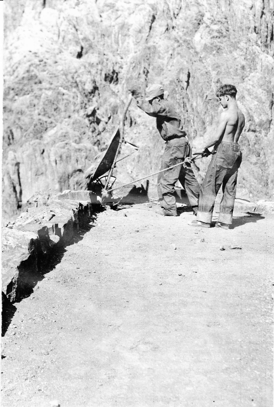
ABOVE: CCC enrollees construct a trail to the Colorado River within the Grand Canyon in 1934.
